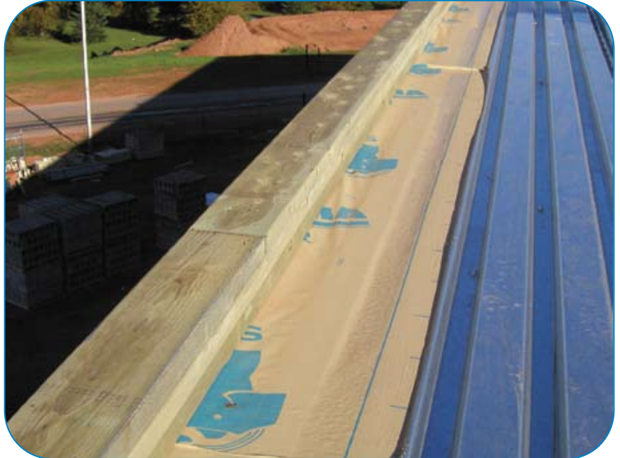
Coordination of the trades to ensure air/vapour barrier continuity is simplified if a self-adhesive barrier is installed by the carpenter before the parapet is constructed.
