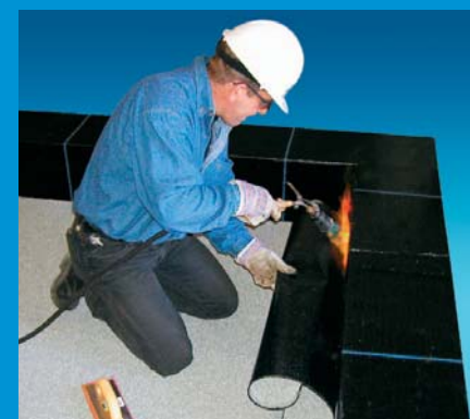
5 Install the cap sheet flashing membrane onto base sheet flashing with torch (or with adhesive).
